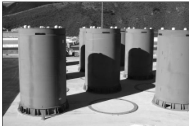
Diablo Canyon Nuclear Power Plant (San Luis Obispo County, CA) irradiated fuel dry cask storage.
