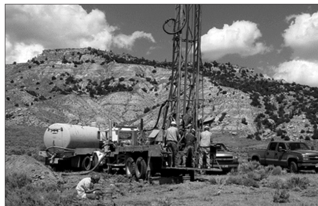
The drill pad is the work site where the rig and other equipment are located, including water supply trucks, drill mud storage tanks, and workers' vehicles. In the foreground a geologist is evaluating "cuttings" laid on the ground after extraction from the borehole.
