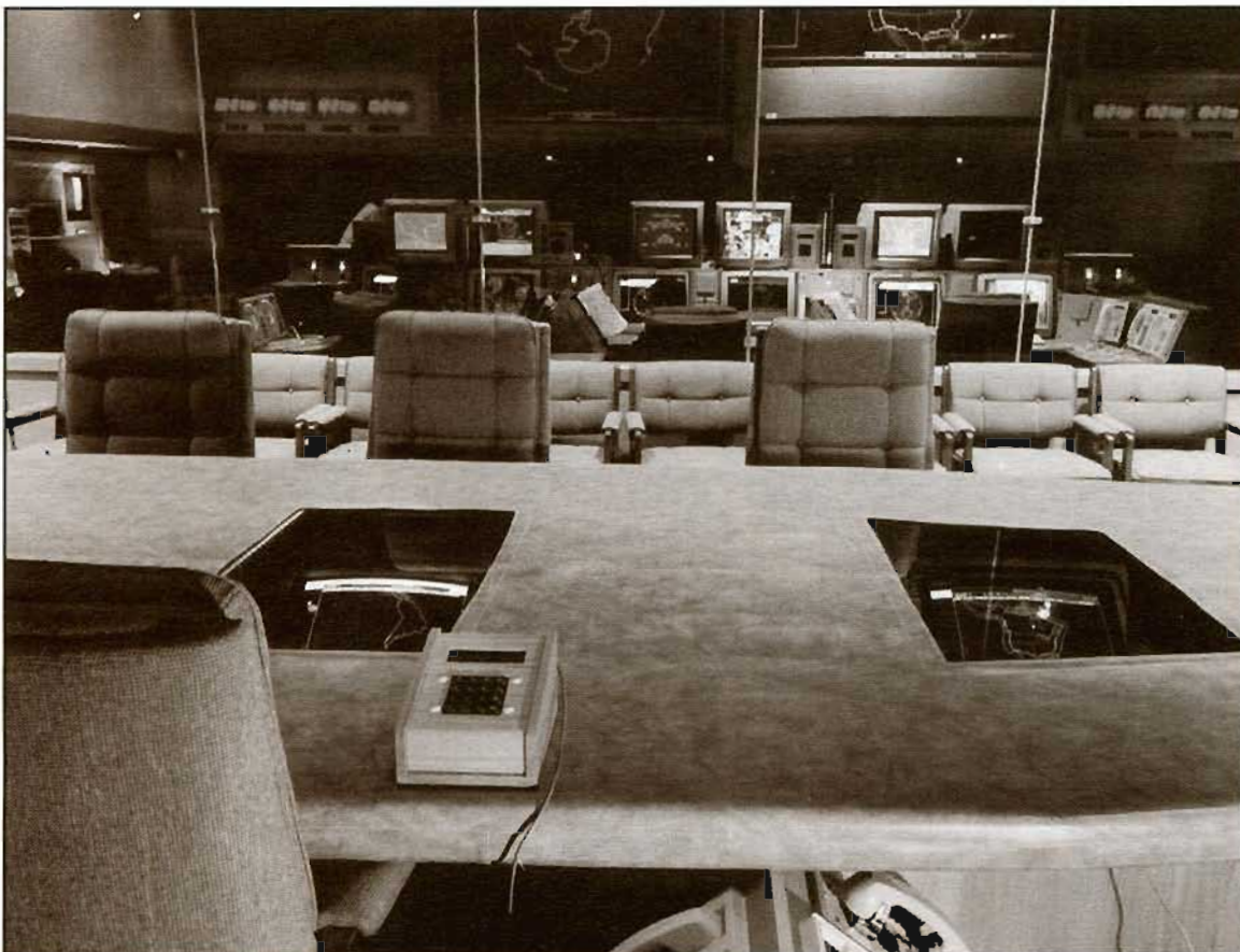
NORAD Commander in Chief's seat in "Battle Cab" - North American Aerospace Defense Command, Cheyenne Mountain Complex, underground attack warning command center, Colorado Springs, CO.
