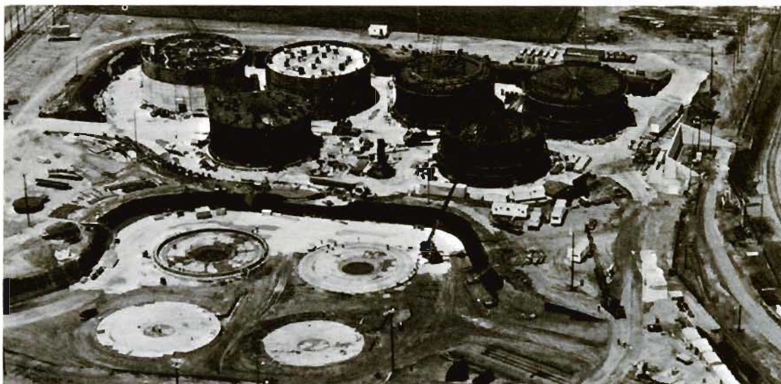
High-level waste storage tanks being built at Savannah River in the early 1980's.
