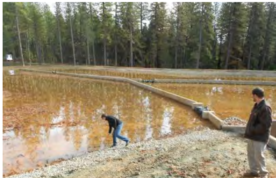
5 - Baffles insure long flow path in Wetland No. 1
