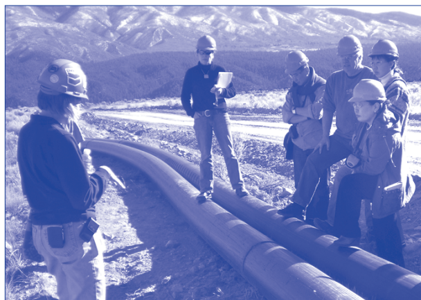
Exchange participants standing on the tailings distribution pipeline at the Chevron molybdenum complex learn about tailings management.
