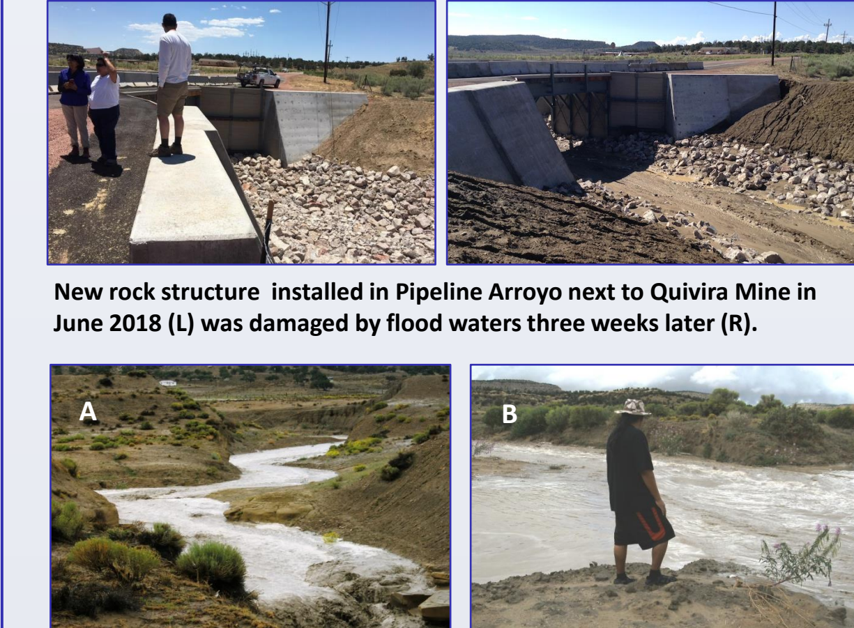
New rock structure installed in Pipeline Arroyo next to Quivira Mine in June 2018 (L) was damaged by flood waters three weeks later (R). Flood waters in Pipeline Arroyo next to the Quivira Mine (A) inundated a crossing on Pipeline Road one-half mile north of the UNC tailings dam in 2012 (B). These points are shown on the 2011 photo montage to the left. (Photo credits top: Paul Robinson, Edith Hood; bottom: Terry Keyanna.)
