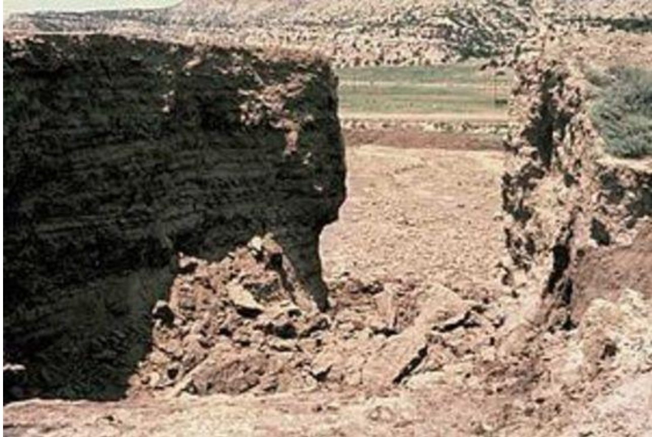
Hole in dam from inside the tailings impoundment SRIC; unknown origin
