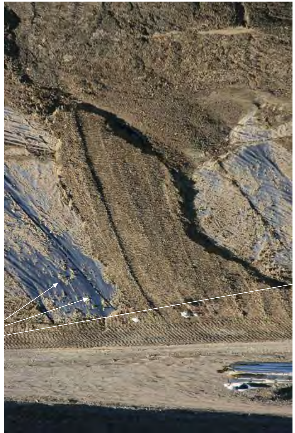
Aginskoe 2007 Liner - Extensive pattern of holes in liner material demonstrates that potential to prevent leaks has been destroyed for this portion of the liner
