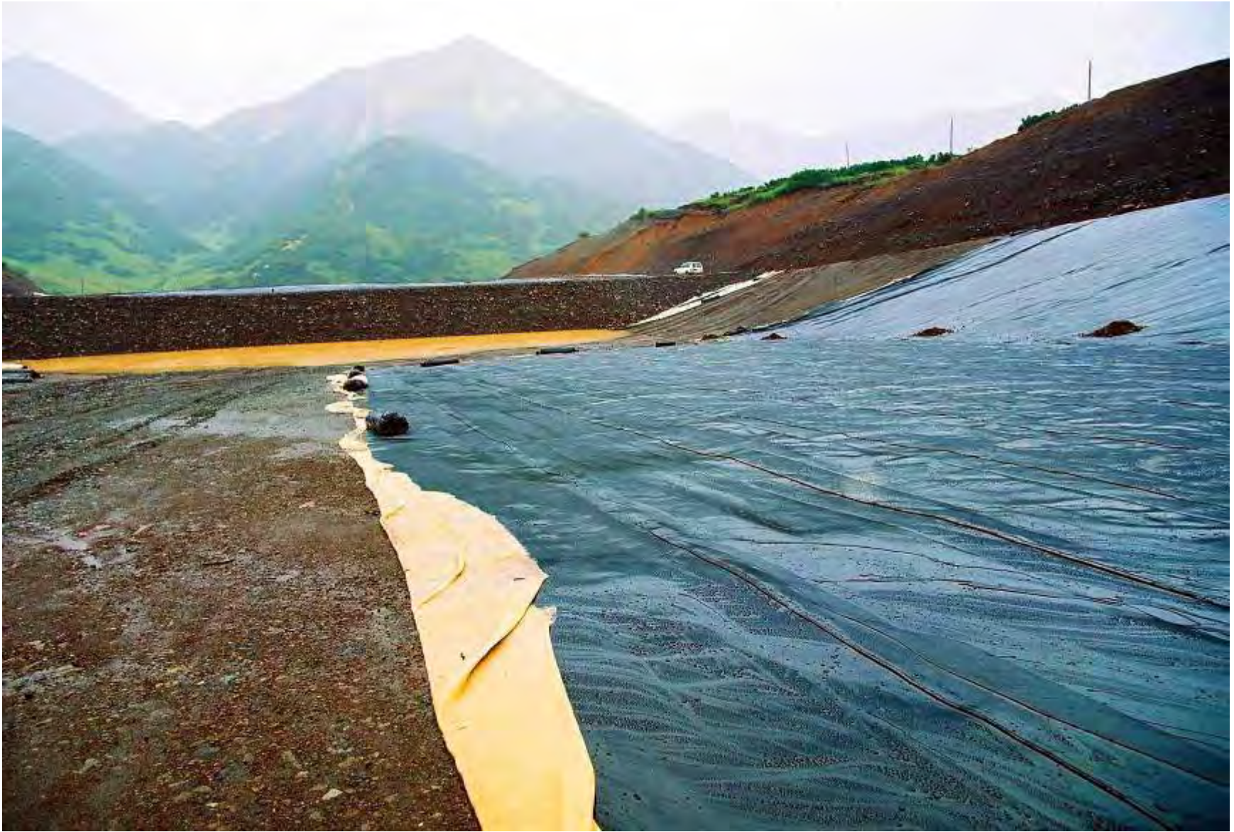
Aginskii Tailings Dam, Kamchatka, Russia, During Liner Installation showing Substrate - “Pillotka” under Liner, Geo-Membrane over Sub-Strate, and Liner Film with Welded Seams - 2005 [Substrate more typically specified as sand rather than pebbles and cobbles]
