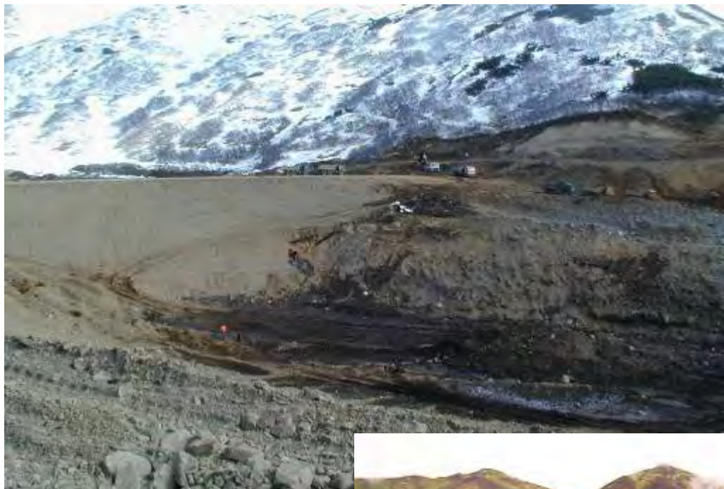
Aginskii Gold Mill Tailings Dam During Slope Construction Before Liner Installation - 2004 - [Note wet zone at base of construction area]
