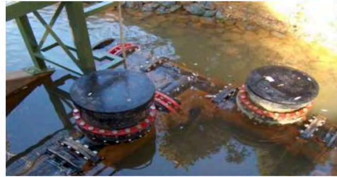
Diversion and Bypass Valves
